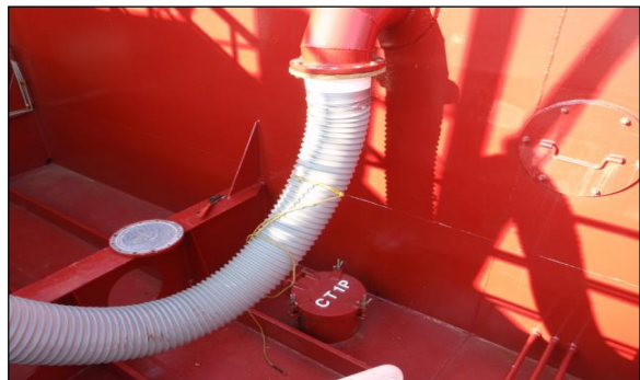
Photo 2. Flex hose to the tank-drying system
