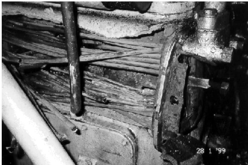
Photo 2. Burst high pressure air cooler tubes and fractured casing.
