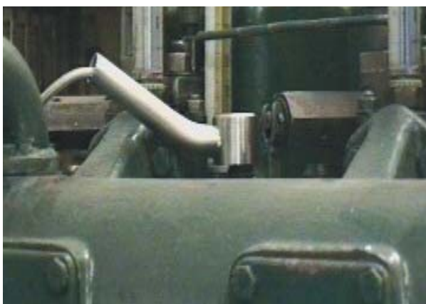
Figure 17: Leakage Measure System onboard in use
